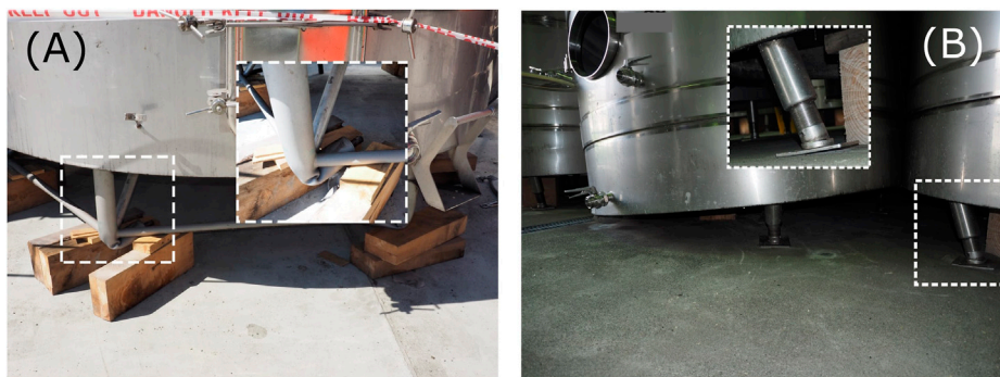
FIGURE 2 Damage on legged tanks: (A) bending of the lower part of the tank legs below the bracing; (B) partial collapse of the base of the tank due to excessive rotation of the tank legs.
