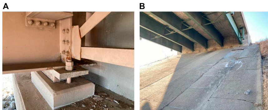
FIGURE 1 Connection between bridge superstructure and abutment of: (A) conventional bridge and (B) integral abutment bridge.
