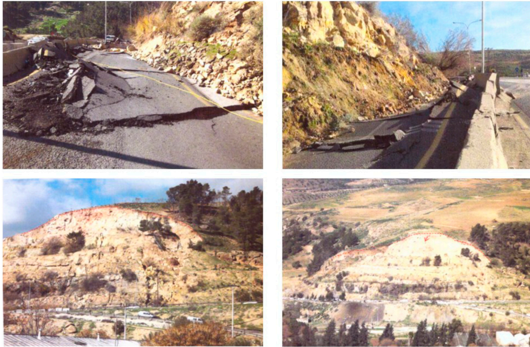
FIGURE 8 | Landslide area at Amman Jerash highway.
