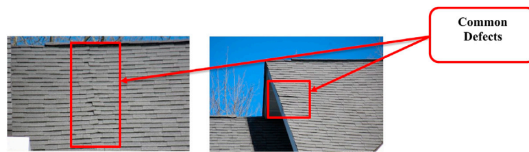
FIGURE 3 Common defects identified on the manually composed aerial images.
