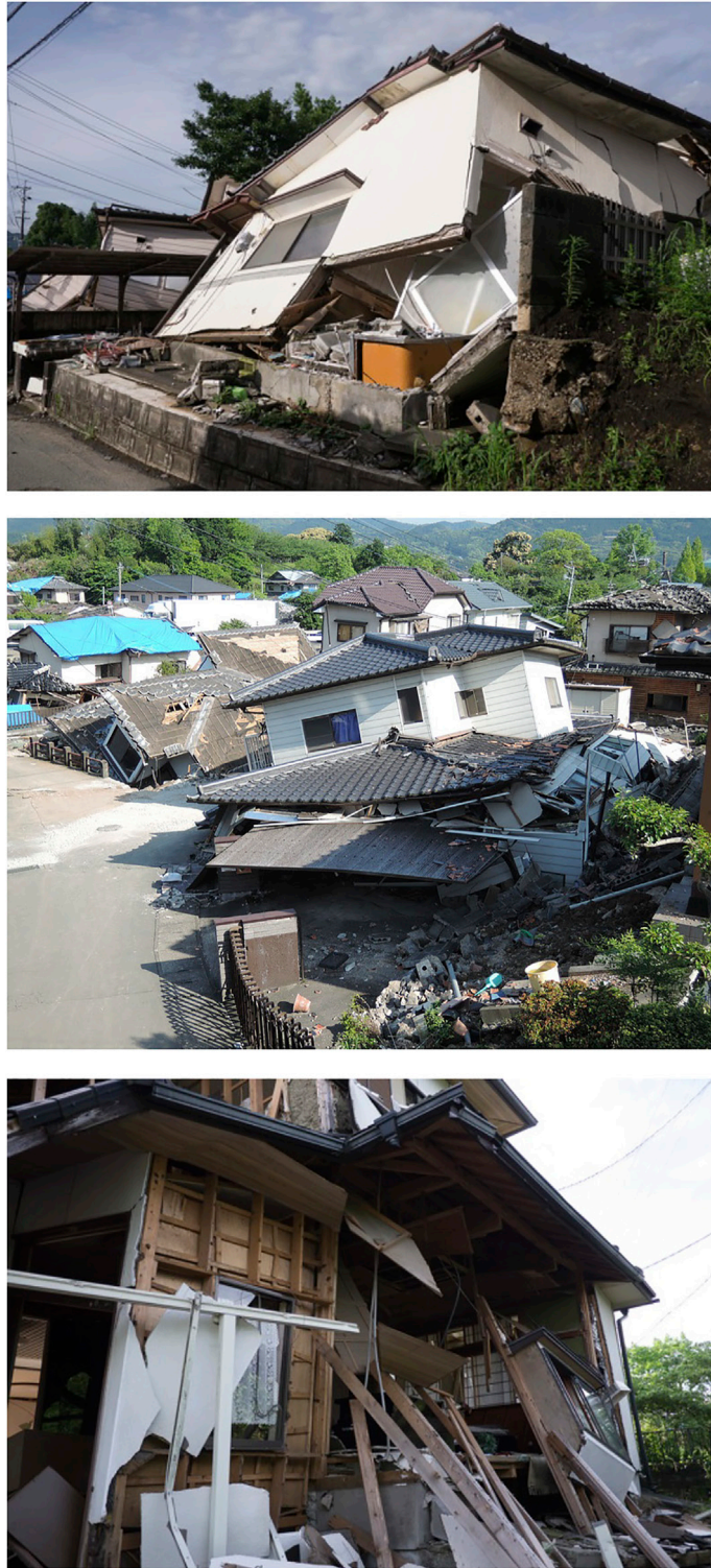
FIGURE 3 | Damage of timber frame houses by the 2016 Kumamoto Earthquake.
