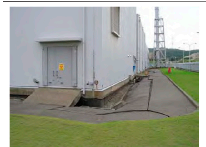
FIGURE 1 | Example of cracks occurring alongside NPP building due to soil settlement below the building (Tokyo Electric Power Company Holdings, Inc., 2007).
