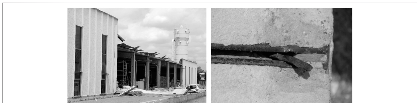
FIGURE 5 | (left) Collapse of concrete cladding panels, and (right) failure of a typical cladding-to-structure connection during the Emilia earthquakes [adopted from Zoubek et al. (2016a)].
