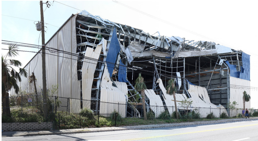
FIGURE 5 | Partially collapsed marine storage building in Panama City, FL.
