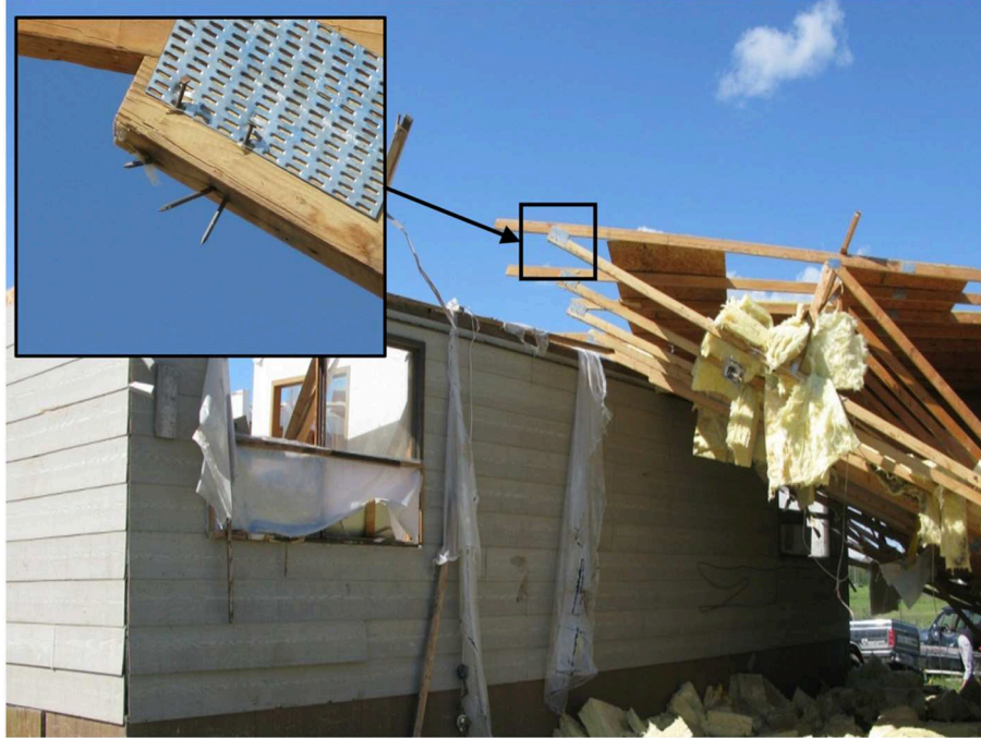
FIGURE 5 | Failure of toe-nailed roof-to-wall connection from an F3 tornado that hit Raymore, SK in June 2010.
