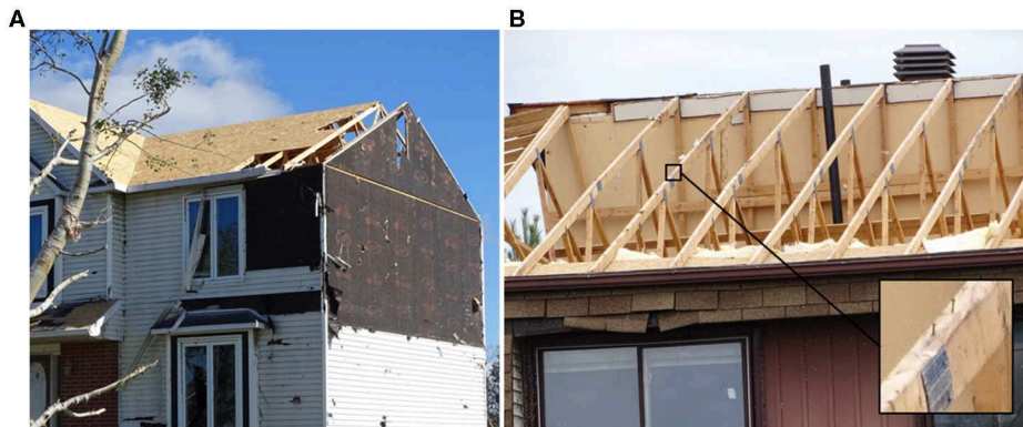
FIGURE 3 | (A) DOD4 sheathing damage (B) Extensive DOD4 sheathing damage showing a magnified example of pull-through failure. Both photos were taken following the Dunrobin, Ontario tornado outbreak of Sept. 21, 2018.
