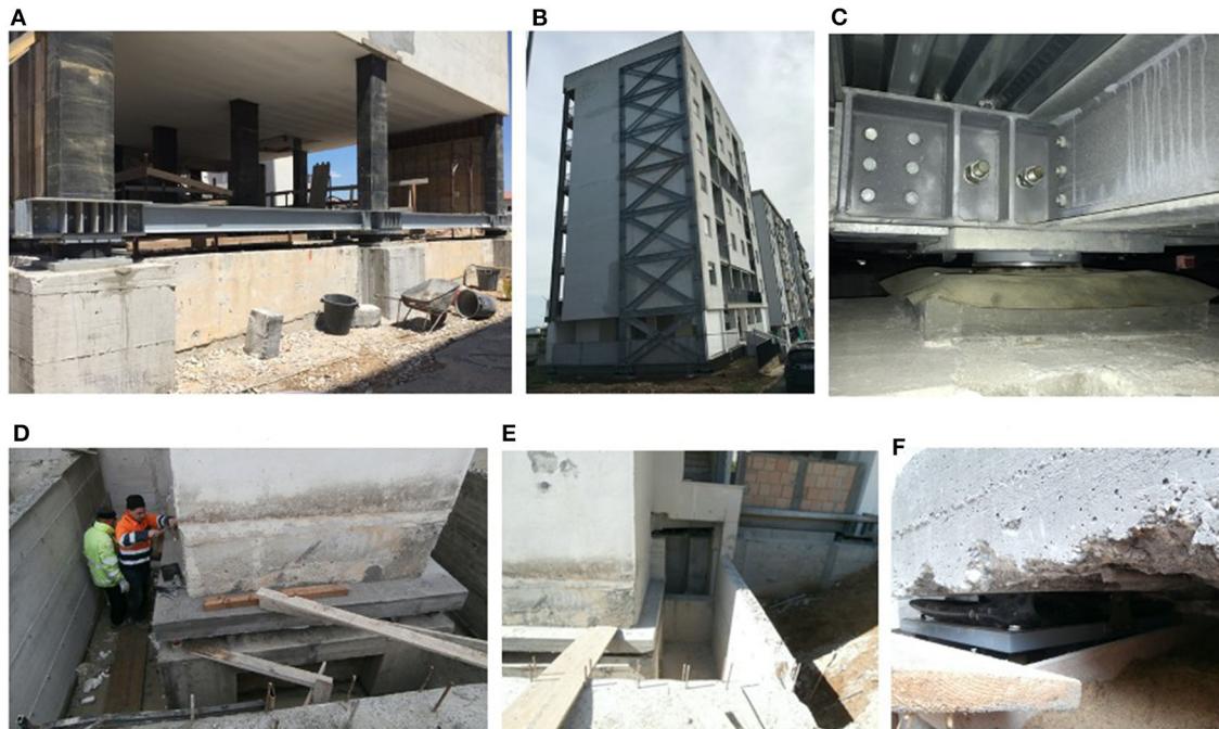
FIGURE 7 | Base-Isolated building. (A) Steel frames grid and seismic device mounted during a construction phase. (B) Lateral view showing the bracing system applied. (C) View a friction slider mounted (view from below the corrugated steel panels). (D,E) Installation of seismic devices under concrete core hosting the elevator. (F) View of the friction slider mounted under a vertical wall.
