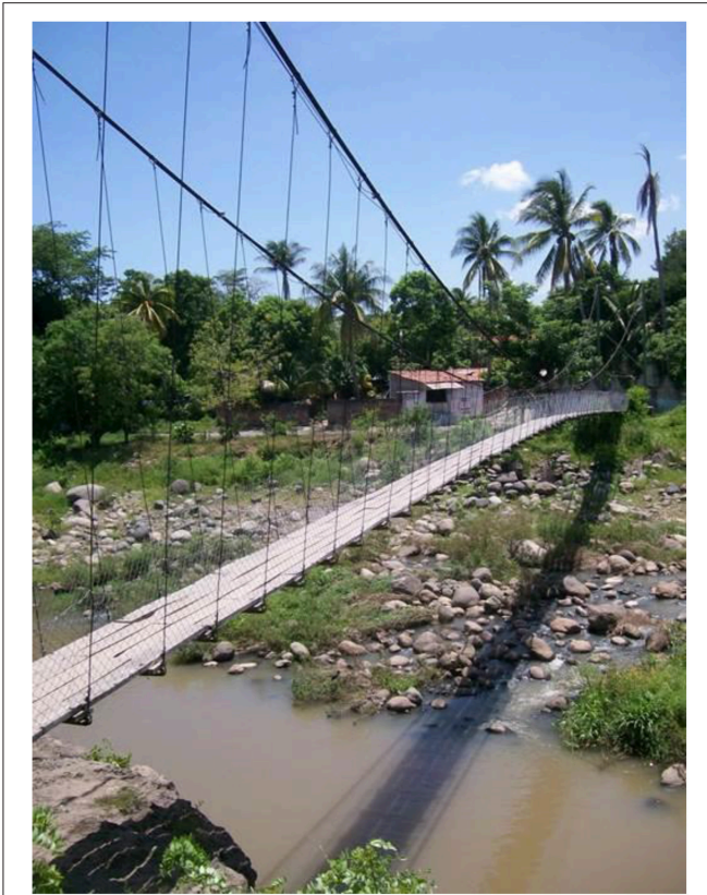
FIGURE 1 | An example of rural footbridge: Melara Footbridge, El Salvador (taken by the first author).
