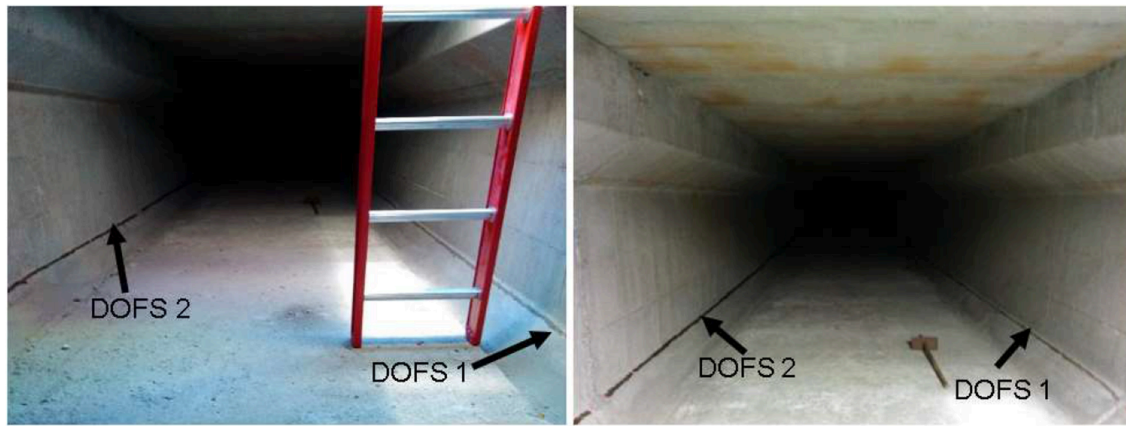
FIGURE 16 | Instrumented DOFS in interior of box-girder beam at Sarajevo bridge.
