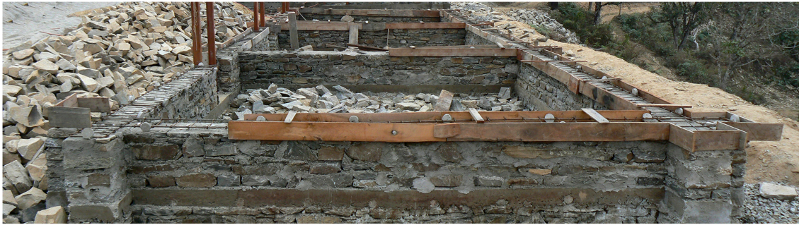
FIGURE 3 | School building in Nepal with rubble stone masonry in cement mortar, brought to courses, and with nominal reinforcements (by courtesy of Smart Shelter Foundation).
