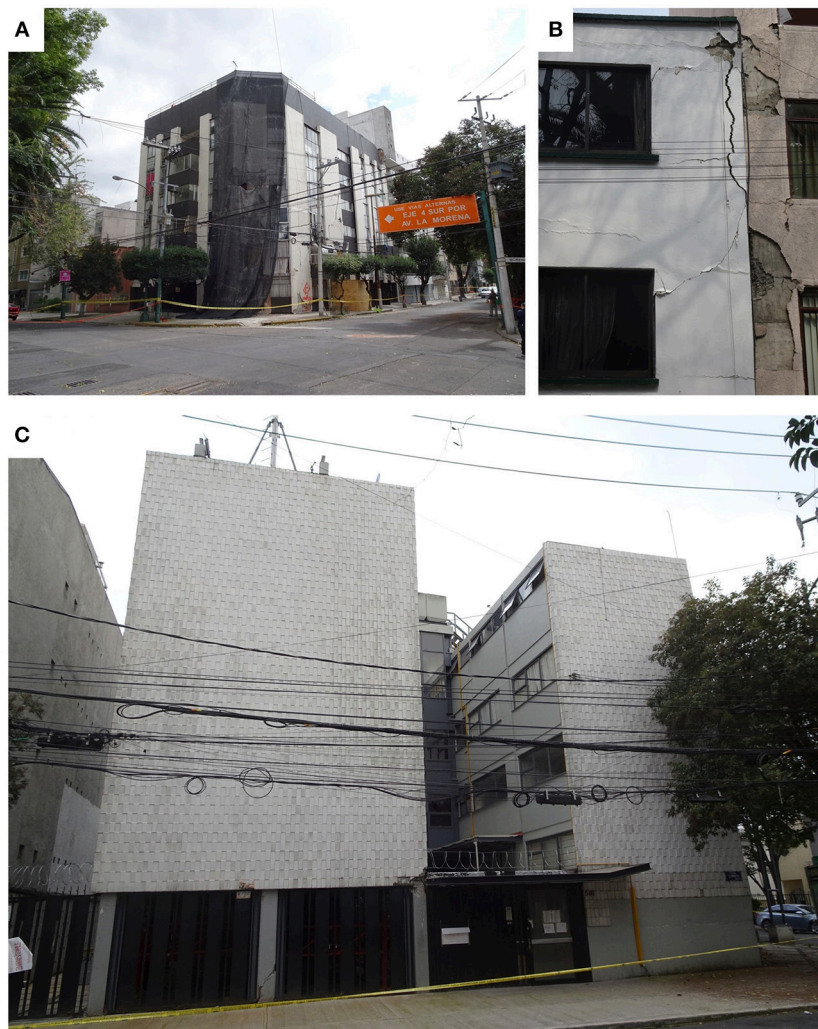
FIGURE 11 | Damage in La Morena. (A) Corner building with torsion eccentricity. (B) Pounding failure. (C) Soft storey in the ground floor.
