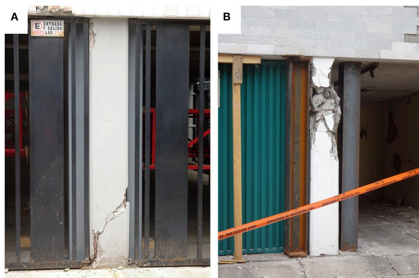
FIGURE 12 | (A) Failure of the column in shear. (B) Buckling of the longitudinal reinforcement bars.
