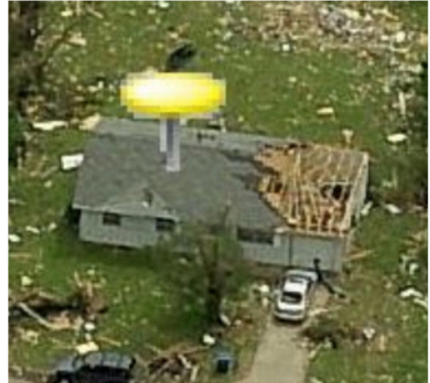
FIGURE 8 | Example of <25% Garage Door Damage, 25–50% Roof Structural Damage. Image resolution and quality reduced for publication. Image courtesy of Eagleview Technologies, Inc.
