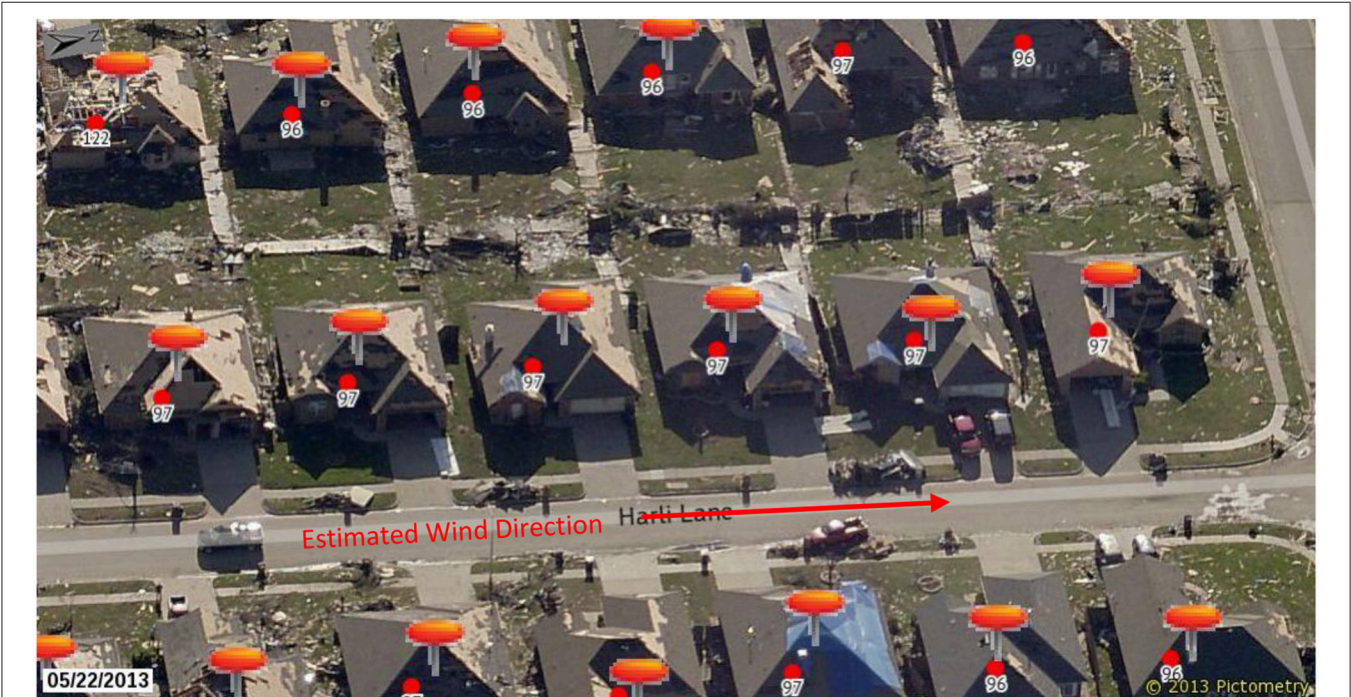
FIGURE 11 | Moore, OK Tornado Damage at Windspeeds Between 90 and 109 mph. Image resolution and quality reduced for publication. Image courtesy of Eagleview Technologies, Inc.
