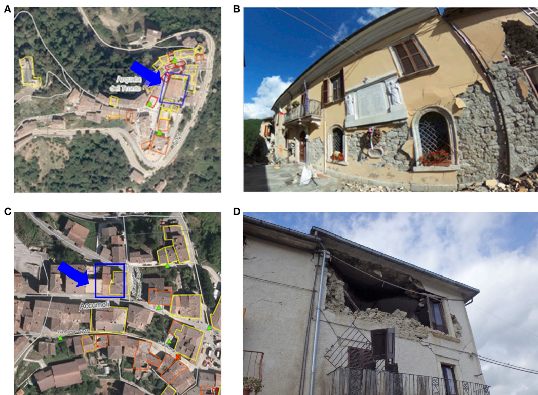
FIGURE 12 | Arquata del Tronto (A) aerial view of the City Hall Building from Copernicus; (B) photographic record. Accumoli (C) aerial view of residential building from Copernicus; (D) photographic record. Copyright: 2016 Copernicus Emergency Management Service.
