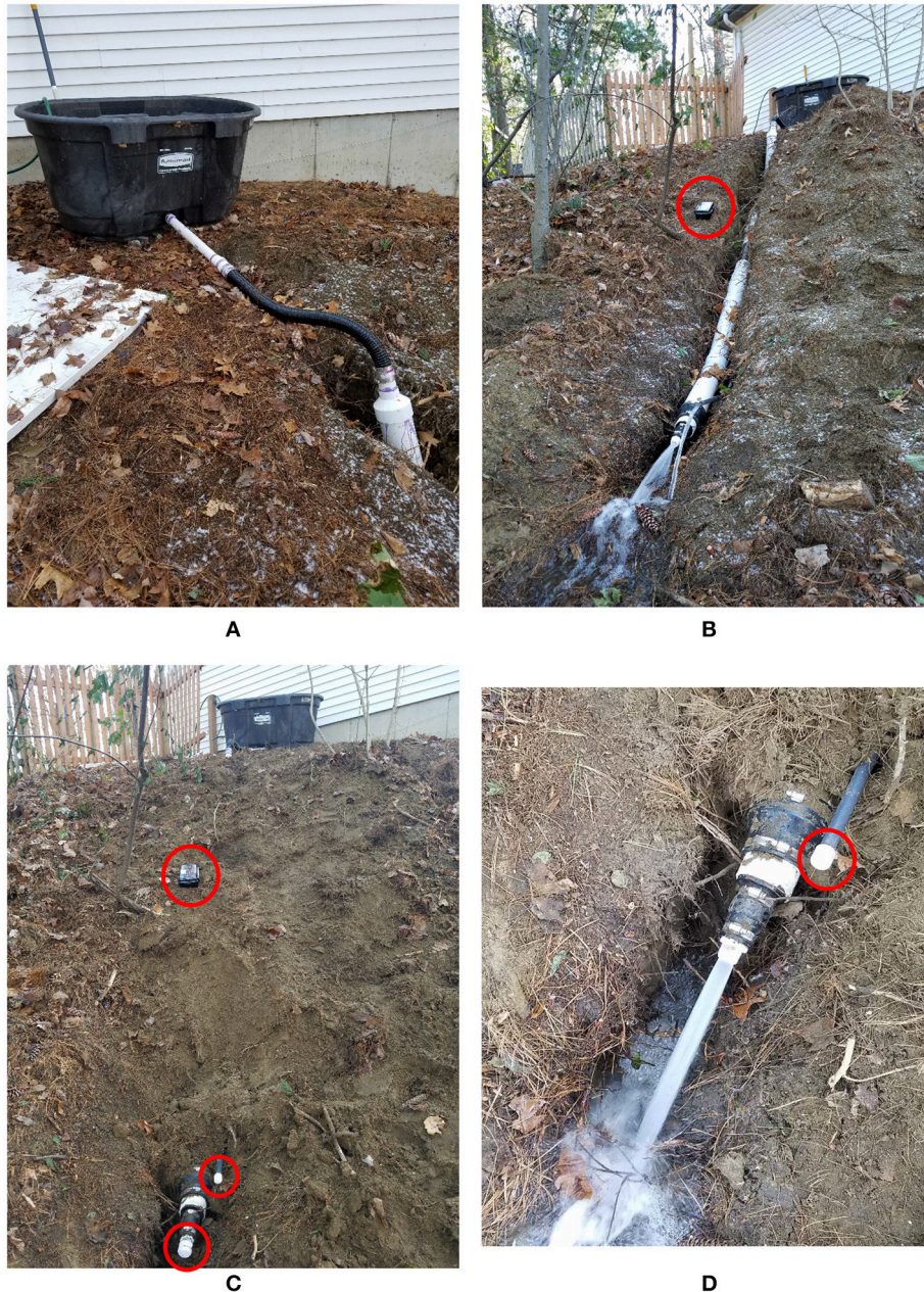
FIGURE 18 | (A) Rain barrel water source for buried pipe containing rotating magnet flow meter. (B) Pipe containing rotating magnet flow meter before burial. Arduino Mega unit with magnetometer and LoRa transmitter is indicated. (C) Pipe after burial. The Arduino Mega unit and the pipe's two drain outlets are circled in red. (D) Water drains through the larger of the two drain outlets. The smaller drain outlet is circled in red.
