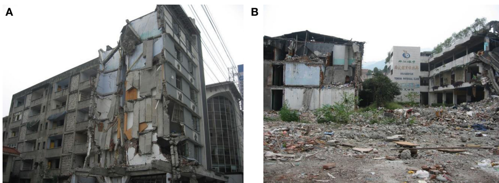
FIGURE 4 | Examples of damaged and collapsed buildings. (A) Typical damaged reinforced concrete building and (B) collapsed and damaged buildings.
