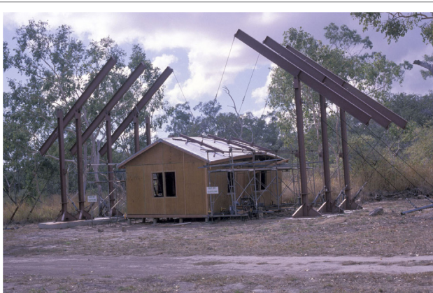
FIGURE 3 | Tongan house after low-cycle failure of truss-to-wall connection.
