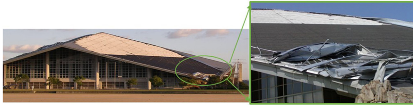
FIGURE 6 | Damage to steel roof sheets on a gymnasium in Kagawa, Japan, caused by Typhoons Dianmu, Namtheun, and Tokage, 2004 [courtesy of F. Nagao and H. Nishimura (Nishimura et al., 2005)].
