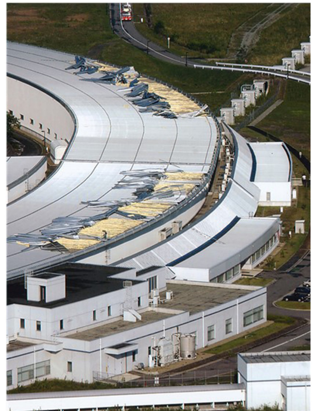
FIGURE 4 | Damage to two-layer folded steel plate roofing system of SPring-8, Riken, Hyogo, Japan, by Typhoon Chaba and Typhoon Songda, 2004 (by Kyodo: Tamura et al., 2005).
