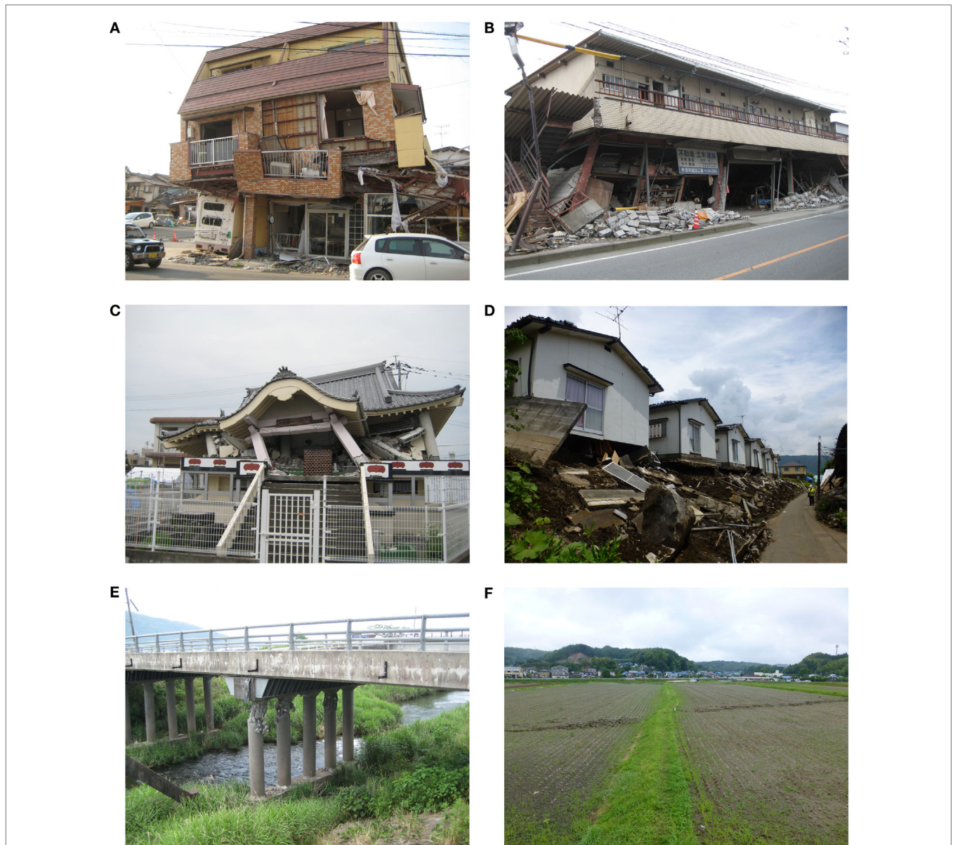
FIGURE 13 | (A) Collapsed steel building along Road 28 (location 5 in region 2). (B) Collapsed steel building along road 28 (location 5 in region 2). (C) Collapsed RC temple near the Mashiki town office (location 5 in region 2). (D) Building damage due to foundation failures (location 5 in region 2; near KMMH16). (E) Failures of RC piers of Daiichi Hatanaka bridge (location 5 in region 2). (F) Fault surface rupture (location 6 in region 2).
