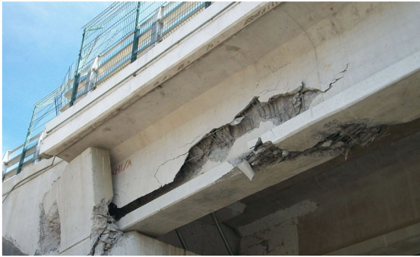
FIGURE 1 | Relative movement induced damage due to the 2010 Chile earthquake.
