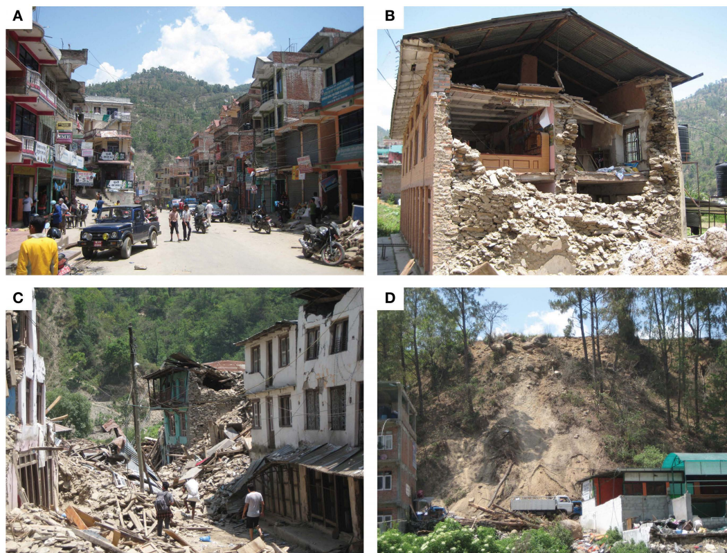
FIGURE 10 | Damage in Melamchi (see Figure 3). (A) Main street in Melamchi. (B) Damaged stone masonry house. (C) Devastated street in Melamchi. (D) Shallow landslide along the main road.
