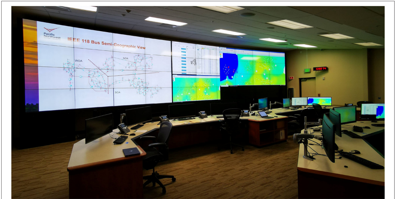
FIGURE 1 | A photo of the electricity infrastructure operations center (EIOC) west control room at Pacific Northwest National Laboratory (PNNL). On screen are a geographical schematic of the IEEE 118 Bus network, several instances of the PowerWorld Simulator, and the ACAT recommender.
