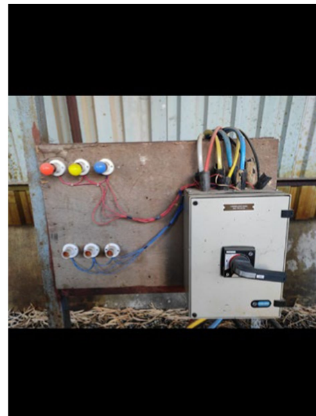
FIGURE 9 Power Discom main supply line.
