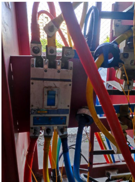
FIGURE 7 Current transformer to main line.
