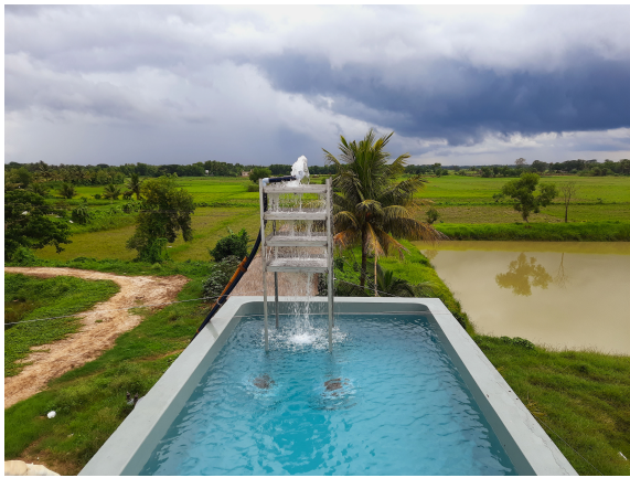
FIGURE 2 Aeration tower installed in the overhead water reservoir tank.
