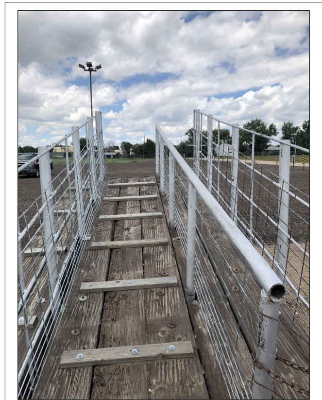
FIGURE 2 | Truck loading ramp for cattle that has cleats (battens) that are spaced too far apart. This will cause the hooves to slip. The cleats should be spaced so that an animal's hoof can easily fit between them. The addition of solid sides would prevent animals from seeing vehicles out in the parking lot. This may also improve animal movement.
