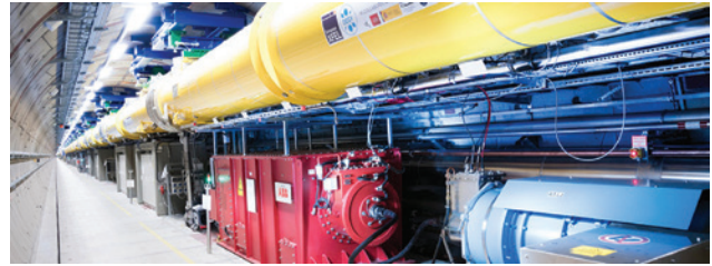
The linear accelerator of the European XFEL is the longest superconducting linear accelerator in the world. It drives electrons up to 17.5 GeV energy (Copyright European XFEL).
