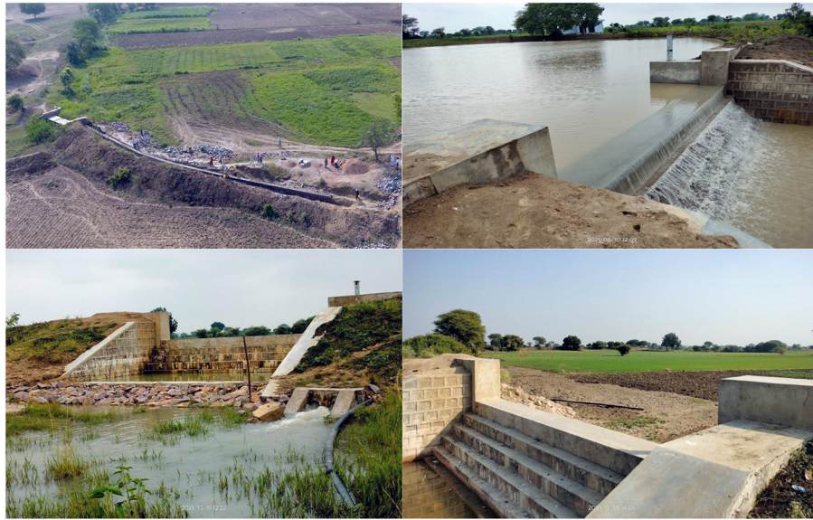
FIGURE 2 | Construction of masonry core wall and spillway (top left); Harvested rainwater in haveli structure during monsoon period (top right); draining out water from haveli before post-monsoon crop (bottom left); wheat crop cultivated on haveli bed during post-monsoon season (bottom right).
