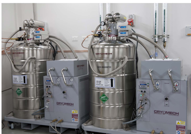
FIGURE 3 - These machines squash and cool the helium gas until it becomes a liquid again.
