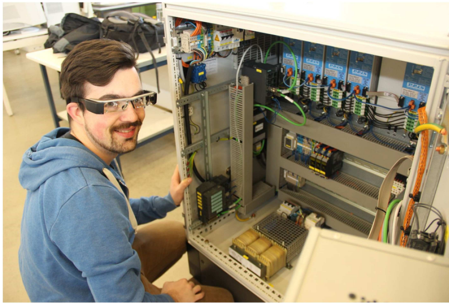
FIGURE 2 | The switch cabinet with integrated servo amplifiers (blue).
