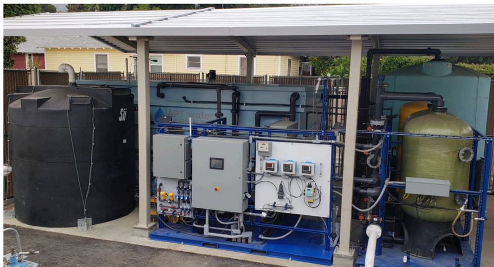
FIGURE 5 | ARoNite™ System in La Crescenta, California.
