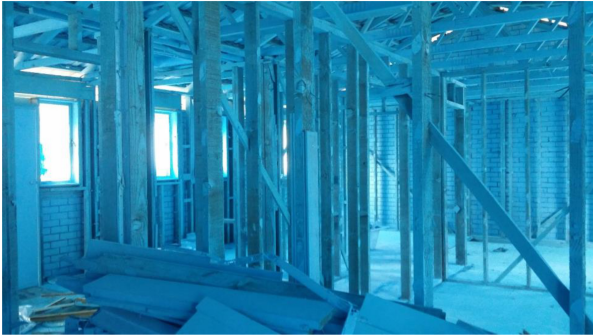
FIGURE 4 | A decontaminated Mr Fluffy home sprayed with a mixture of PVA and blue paint to bind any remaining loose fibres prior to removal to landfill.
