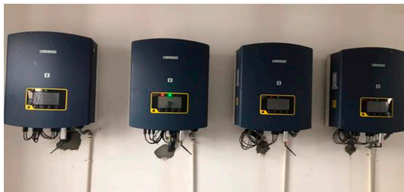
FIGURE 3 Hardware setup of the inverters.
