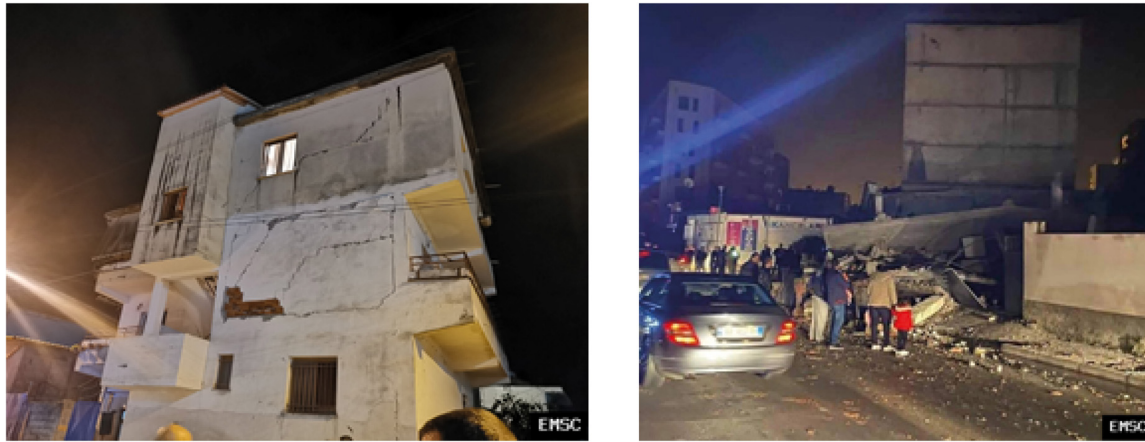
FIGURE 7 | The first crowdsourced picture exhibiting structural damage (left) was collected 64 min after the mainshock and located in Tirana, 30 km from epicenter. The first collapse (right) was collected 77 min after the mainshock and taken in Durres, less than 10 km from the epicenter.
