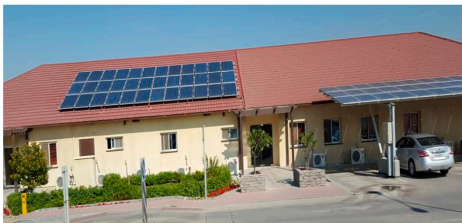
FIGURE 2 The second 8.64 kW PV installation on a building in Bahrain (Sadeem building) in Awali in 2014 by Bapco. There are 36 PV rooftop panels, each having 240 W p (Alnaser, 2017; Alnaser and Alnaser, 2017).
