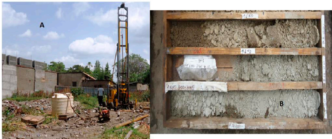
FIGURE 3 (A) Field investigations and excavation (B) SPT samples and wooden core boxes.
