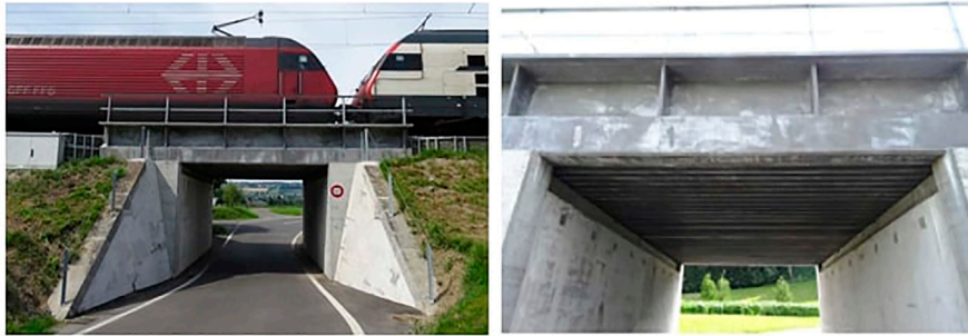
FIGURE 13 | Railway underpass Unterwalden (Sempach) with a structure in R-UHPFRC resting on concrete abutments. (Photographs: E. Brühwiler).
