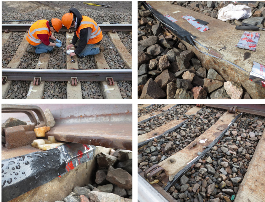
FIGURE 2 | Images of sleepers instrumented with concrete surface strain gauges at a HAL freight railroad field experimentation location.
