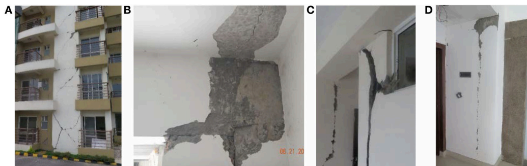
FIGURE 2 | Observed damage on different components of the building. (A) Exterior damage. (B) Beam-column joint. (C) Interior infill wall. (D) Separation between column and infill.
